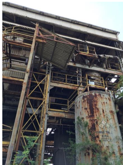
Inside view of the rusted Storage Tank E. H. 4 (not for MIC)
